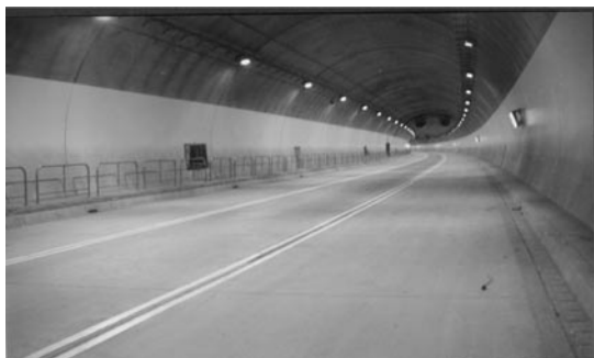
Figure 3-1 Longitudinal Lighting System
